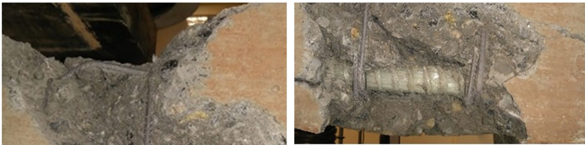
Figure 12. a Crushed concrete. b. Intact GFRP bars.
