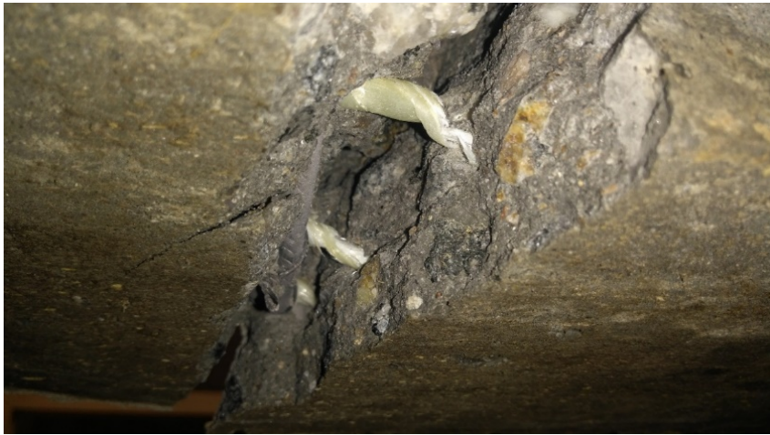
Figure 7. Rupture of the GFRP bars of the VV23.
