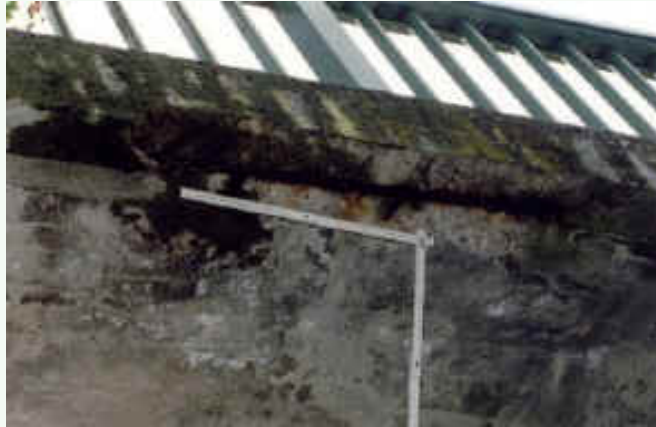
Steel corrosion of the bridge cap (deicing salt, sea water environment)
