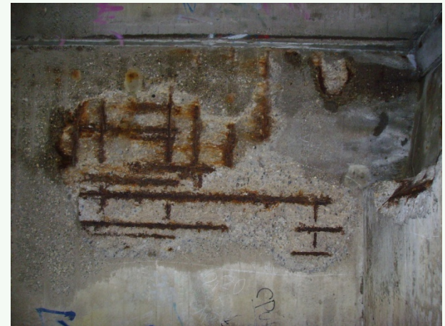
Corrosion due to less concrete cover
