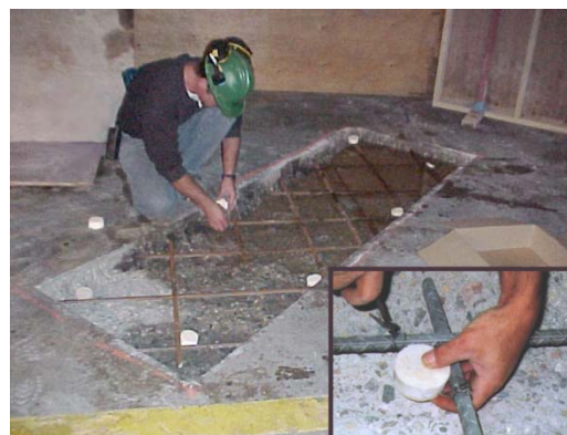
Figure 2: Alkali-Activated Discrete Galvanic Anode Installed For Localized Protection Around Concrete Patch Repair
