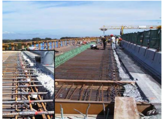
Figure 3: Discrete Anodes Used for Bridge Widening at the Interface Between Old and New Concrete
