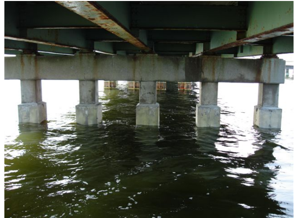
Figure 12: Completed Pile Repair (Galvanic Encasement with FRP Jacket) for New York State DOT
