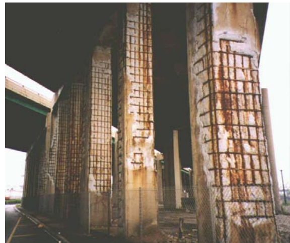
Figure 1: Bridge Columns Damaged by Corrosion of Reinforcing Steel Due to De-icing Chemical Exposure
