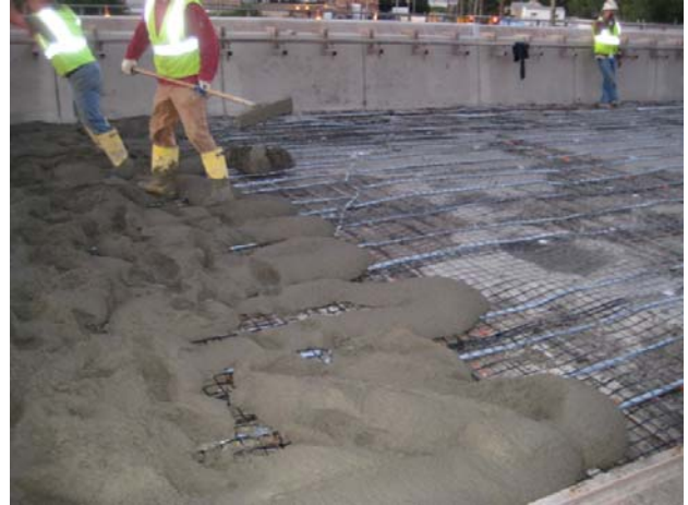
Figure 10: Concrete Overlay Placement over Distributed Galvanic Anodes on Ohio DOT Bridge Deck
