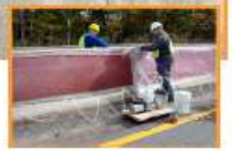
Pavement joint damage on an ASR-affected pavement near Mountain Home, ID (top); Vacuum impregnation treatment on ASR-affected highway barriers near Leominster, MA
