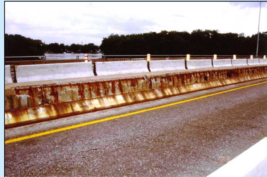
Vachon Bridge, Laval, Canada, 1996 (before rehabilitation, after 22 years of service)
