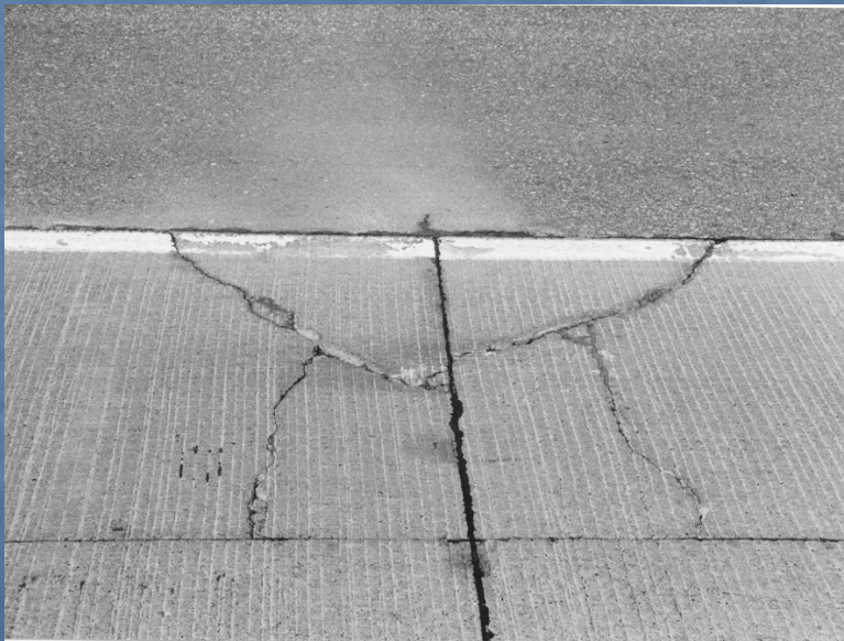
Corner Breaks & Transverse Cracking
