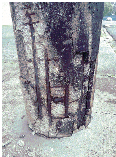
Figure 1 – Reinforcements' corrosion in a reinforced concrete column.
