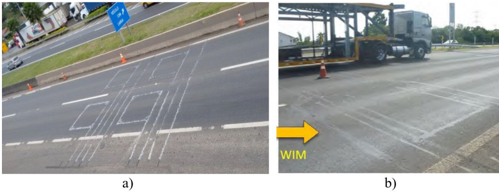
Figure 6. Final appearance of HS-WIM system in both highways: a) BR-381 [15]; b) BR-290 [16].
